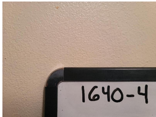
1640-4 Drywall Joint Compound/White (2% Chrysotile) Interior Bathroom Walls
